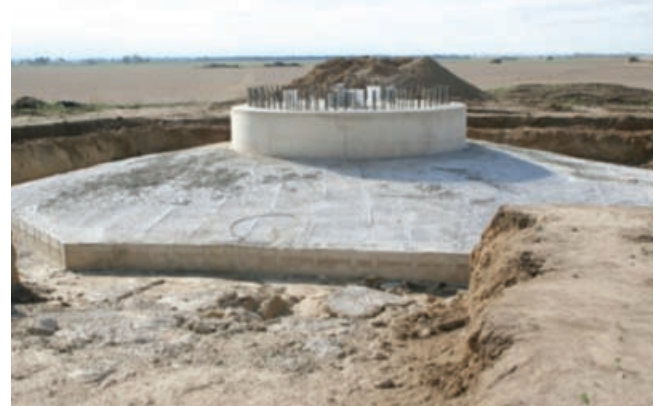
Figure 2. The construction of a utility-scale wind turbine foundation in Benton County, Indiana.
